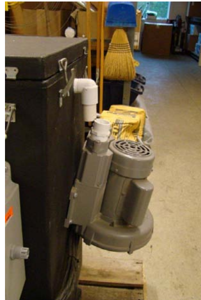
Figure 15 –A Typical wall deformation from air blower on an AirRaider.
