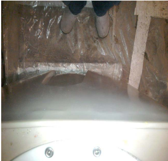
Figure 14 –This picture is view looking down from the top of a Bubble-Up that has only been installed for a few months. This surface is supposed to be straight.
