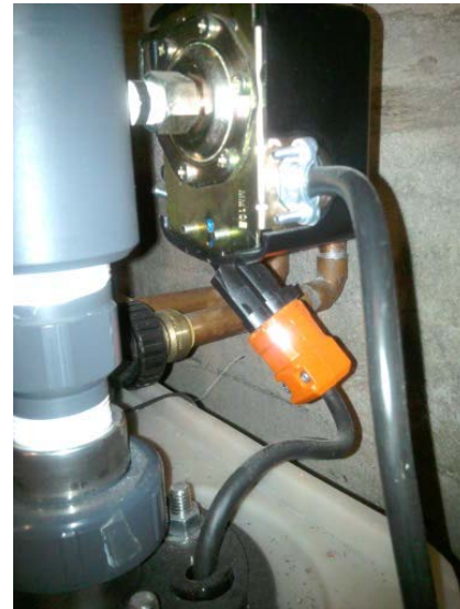
Figure 13 - Bubble-Up shown with a standard low pressure cut out switch for pump protection which is unreliable and is difficult for the homeowner to reset.
