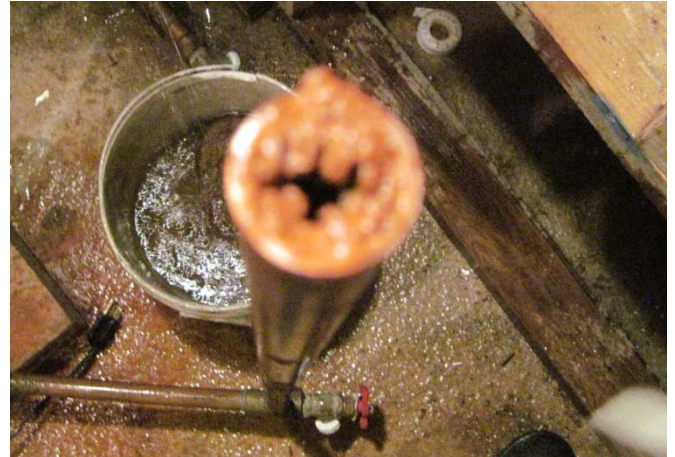
Figure 1- Fouled by air injection system
