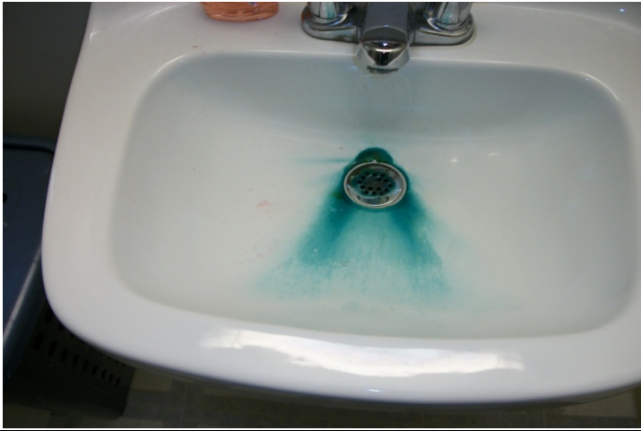
Figure 1 Blue Green Staining from Copper Corrosion
